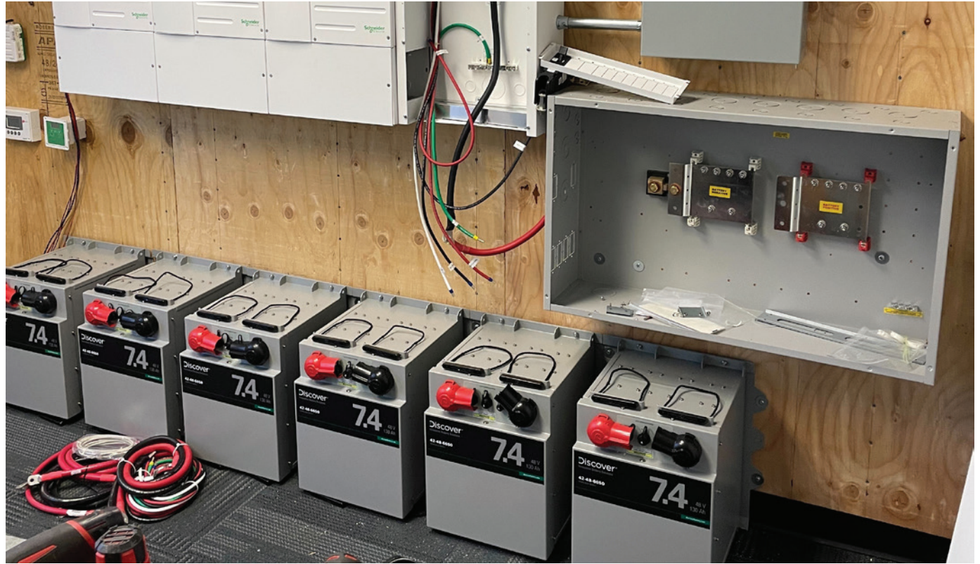
20kW Schneider Inverter System @ 208VAC with 38.4kWh Lithium (LFP) Battery Storage – installed in Thousand Oaks, CA
