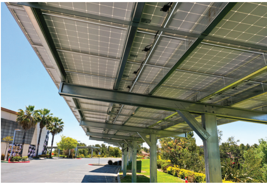
Carport style solar arrays can help increase space available for installation on your commercial property.
